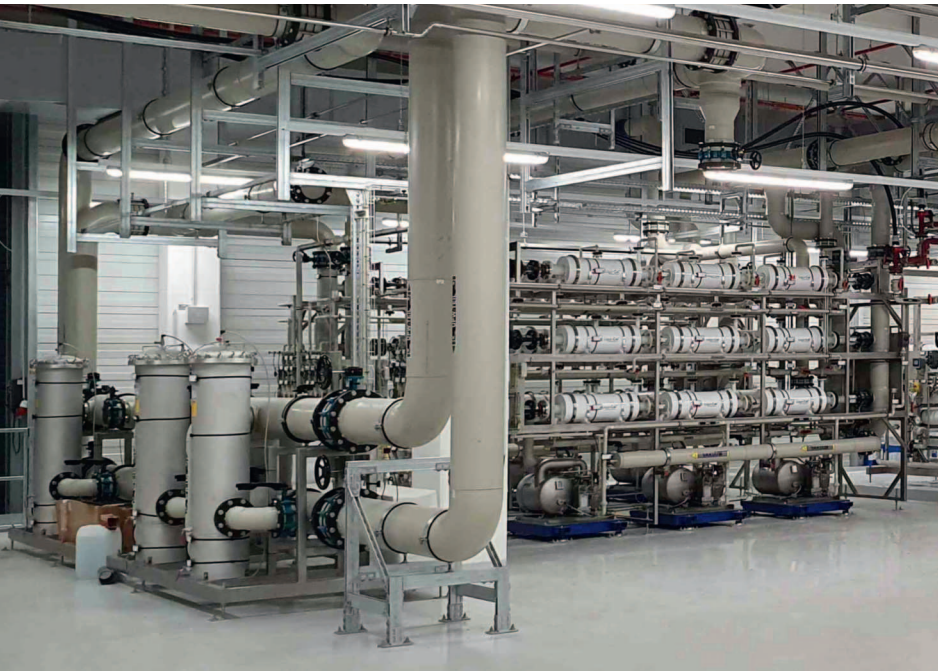
Pre-filter and membrane degasifier
