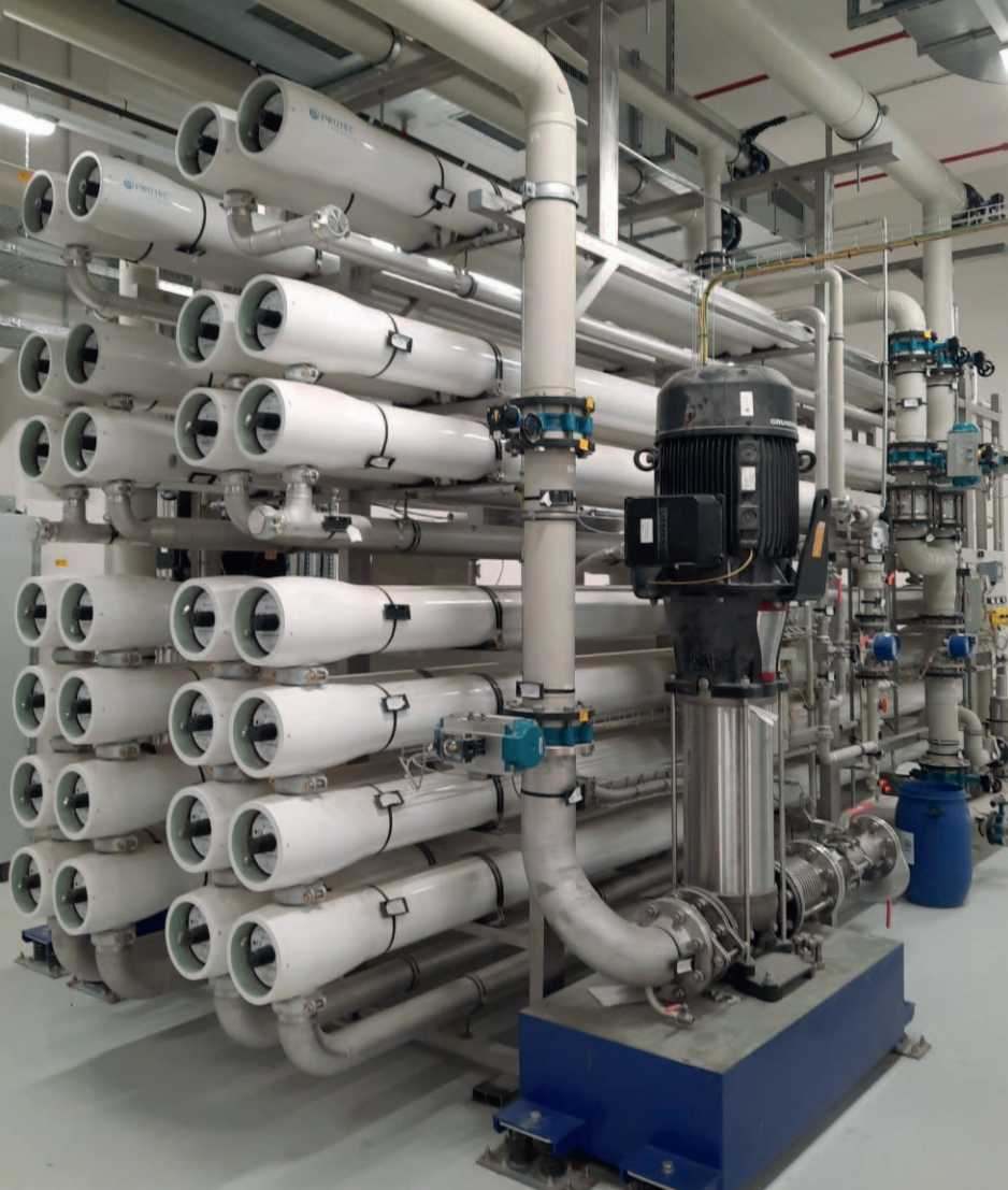
Reverse osmosis plant
