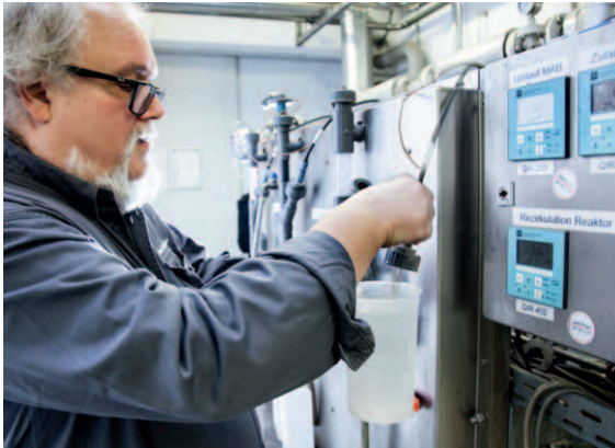
Our service includes all parts of an anaerobic plant.
